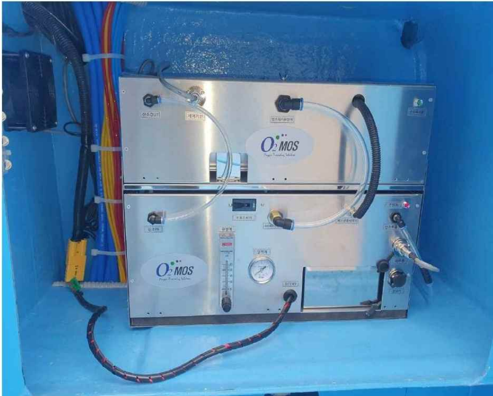
O2MOS unit installed and operating in a live fish transport truck bed.
